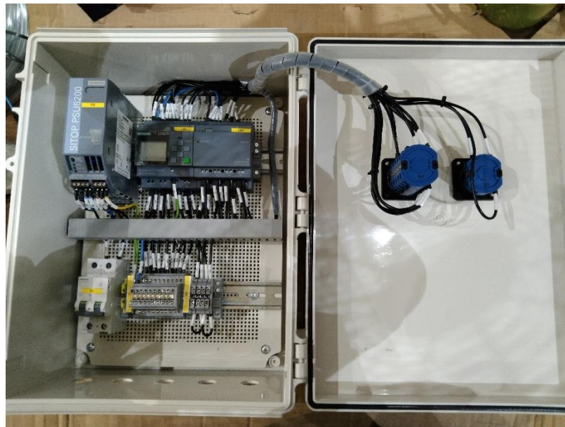
Gambar 2. 1 Panel control PT. Martin Supra Engineering
