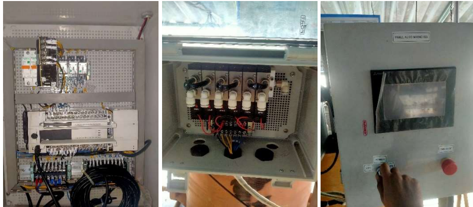
Gambar 4. Wiring Control Panel
