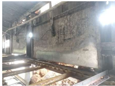
Gambar 2.1. Pintu loading ramp
