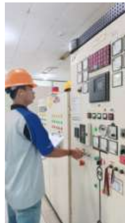
Gambar 2.2 Monitoring panel control generator
