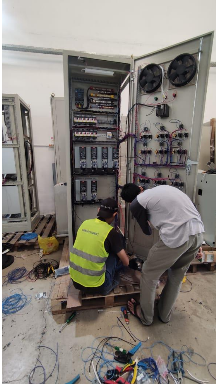
Gambar 2. 23 Panel Kontrol Cooling Tower Fan PT.Rajawali Anugrah Prima
