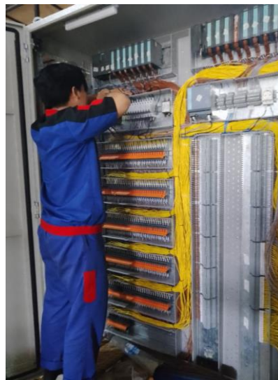
Gambar 2.3 Wiring panel PT. Andalan Furnindo
