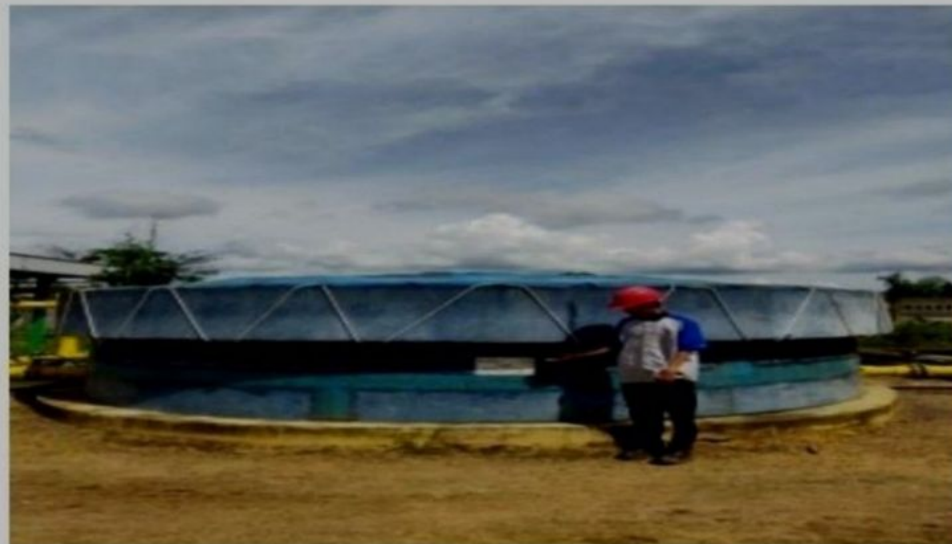
Gambar 1. 12 Dry Biological Filter
