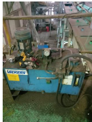
Gambar 2.21 Hydraulic Power Pack
