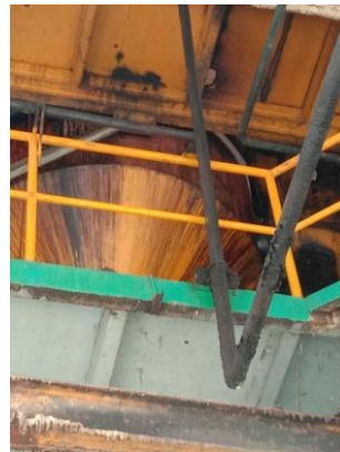
Gambar 2.26.1 Sludge Tank (Tangki Lumpur)
