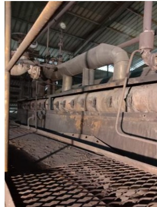
Gambar 2.38 Super Heater Boiler
