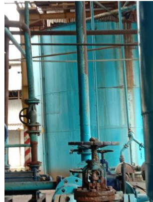
Gambar 2.36 Feed Water tank
