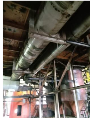
Gambar 2.22 Horizontal Cake Breaker Conveyor (HCBC)
