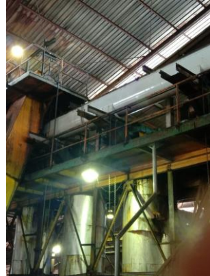
Gambar 2.18 Digester Feed Conveyor
