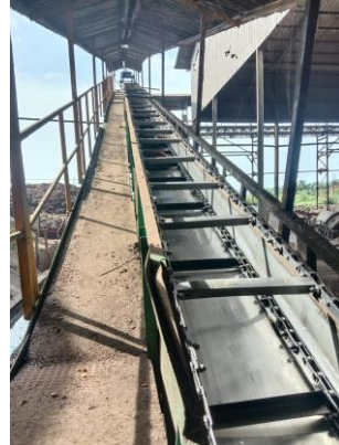
Gambar 2.14 Inclined Empty Bunch Conveyor (IEBC)
