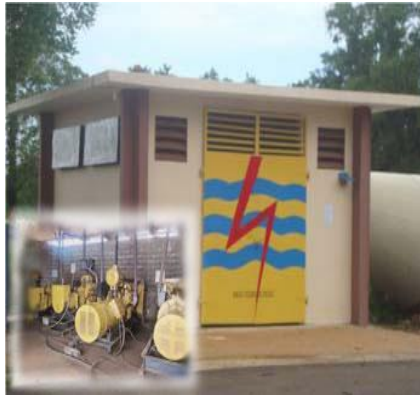
Gambar 1.3 ELECTRICITY ( PLN AND GINSET)
