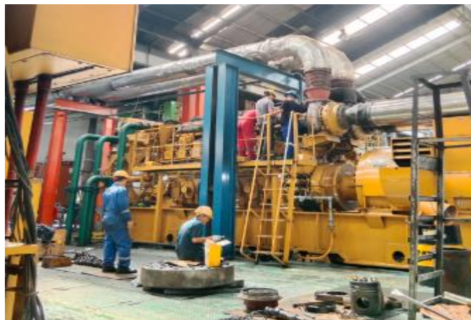
Gambar 2.5 Corrective Maintenance Caterpillar Engine Generator
