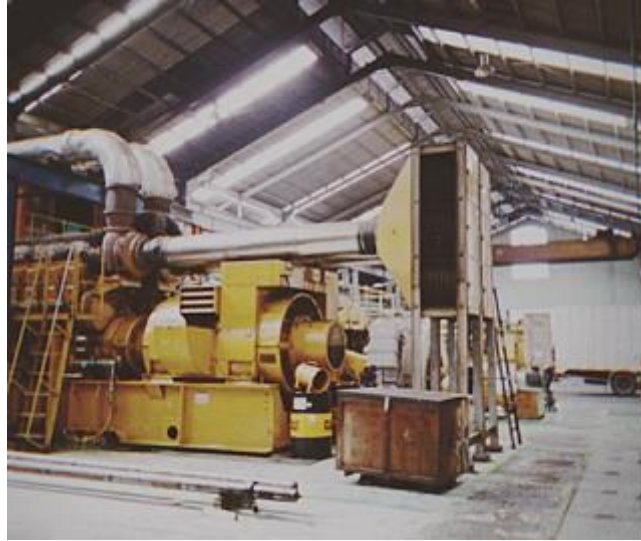
Gambar 2.4 Predictive Maintenance Caterpillar Engine Generator
