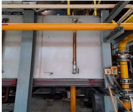
Gambar 1. 28 Clean Oil Tank
