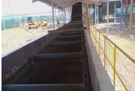
Gambar 2. 2 FFB Inclined Scrapper
