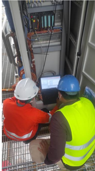
Gambar 2.3 wiring panel PT. Sumber Indahperkasa
