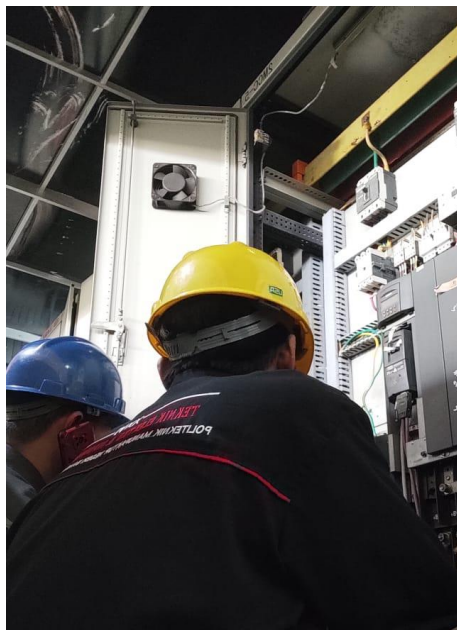
Gambar 2.2 wiring panel PT. Sumber Indahperkasa
