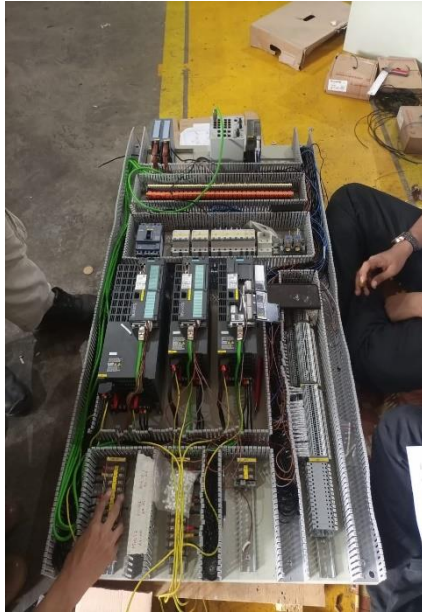
Gambar 2. 1 Terminasi di Panel PLC PT. Firmenich Indonesia
