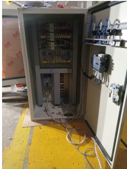
Gambar 2. 3 Terminasi di Panel Distribusi PT. Firmenich Indonesia
