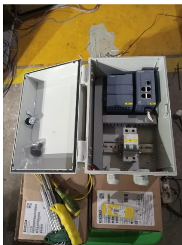
Gambar 2. 4 Terminasi di Panel Repeater PT. Firmenich Indonesia
