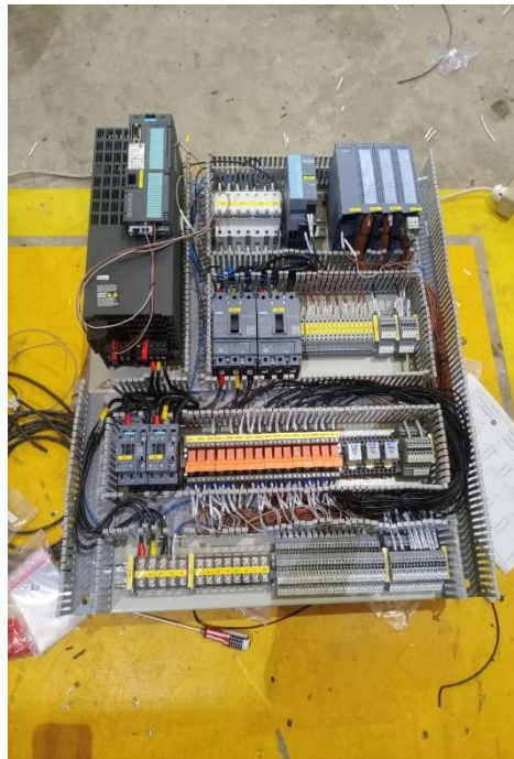
Gambar 2. 2 Terminasi di Panel PG Transfer PT. Firmenich Indonesia
