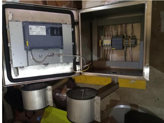
Gambar 2. 5 Terminasi di Panel HMI PT. Firmenich Indonesia
