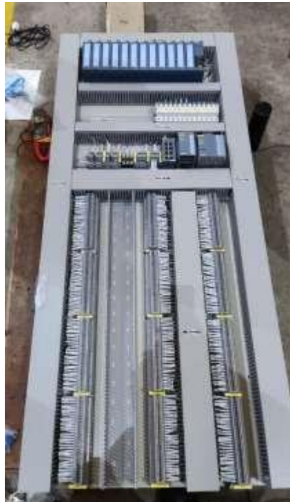
Gambar 2. 14 Panel PLC PT. Pupuk Kujang Cikampek
