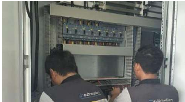
Gambar 1. 24 Control Panel Assy
